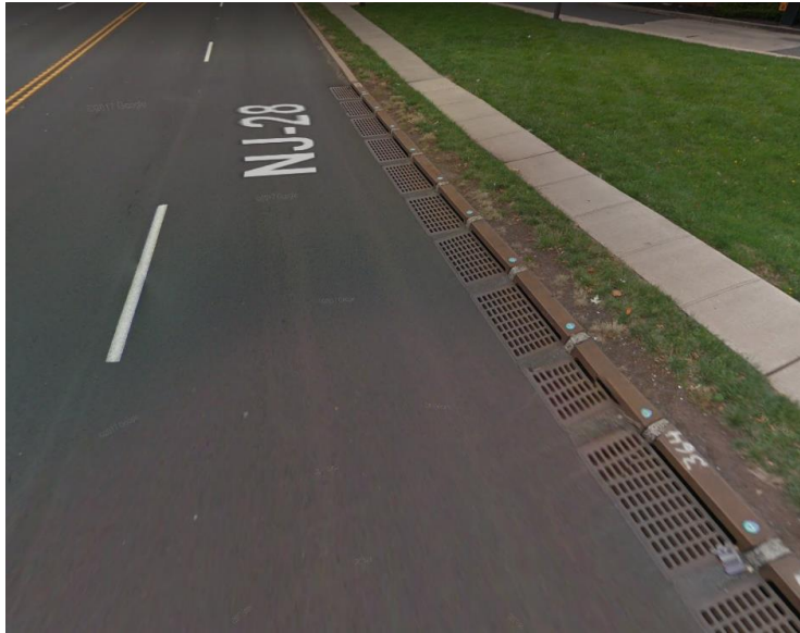
Figure 63. Google Maps Street View image of an example location with a set of inlets to capture extreme events along the road.
