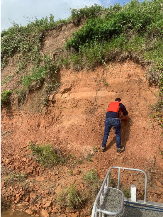
Figure 1-7: Riverbank Erosion just north of the intake pipe for MRPS.
