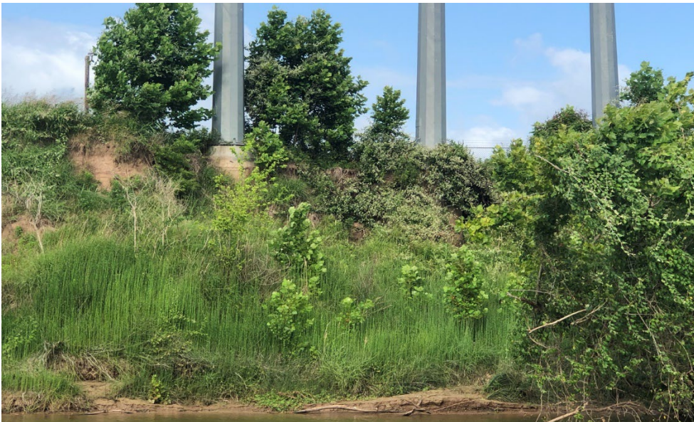
Figure 1-5: Exposed Power Transmission Poles near Mary Rhodes Pump Station (Up-close)
