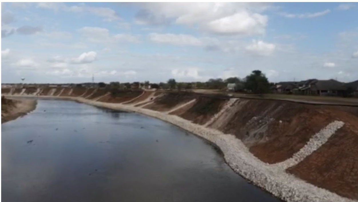
Figure 2-2: Example of Alternative 5 as constructed on the Brazos River near Richmond, TX
