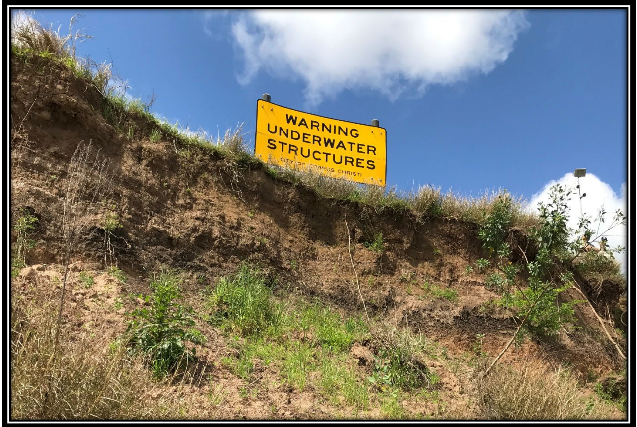
Figure 7 - Photo showing bank erosion at site of the Mary Rhodes Intake
