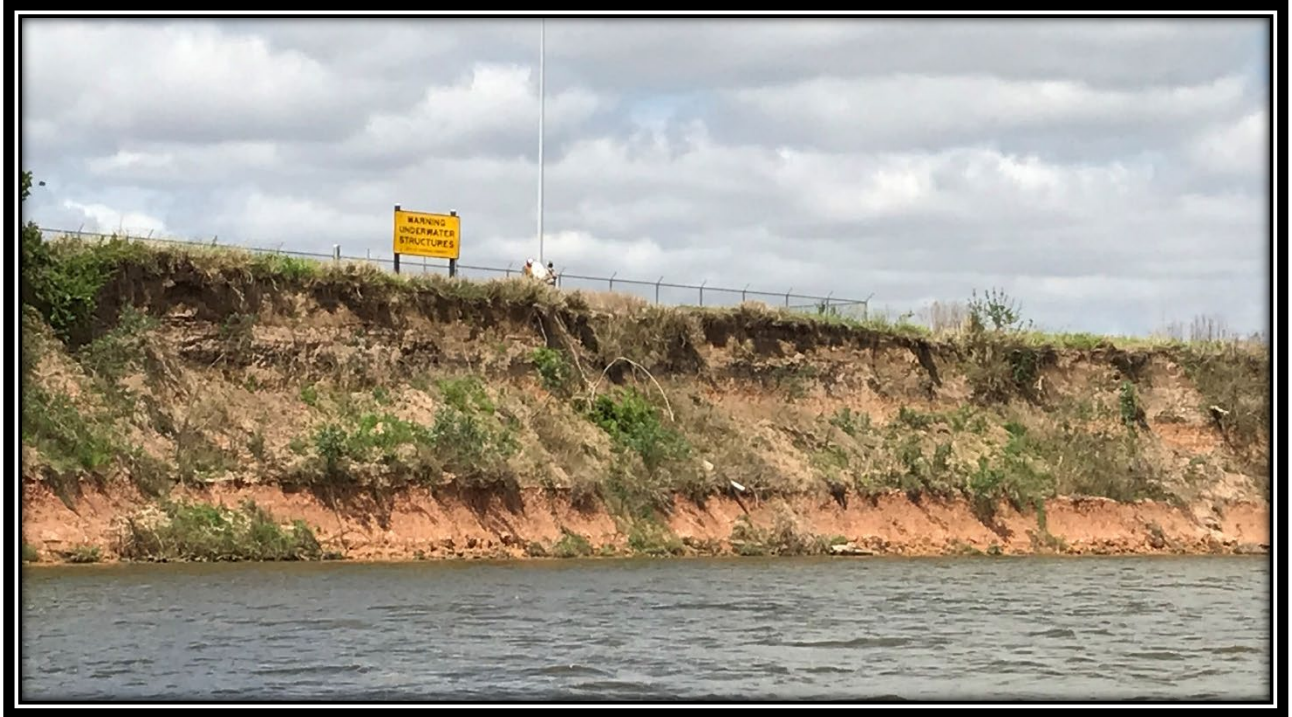
Figure 6 - Photo showing bank erosion encroaching on Mary Rhodes Pump Station Intake
