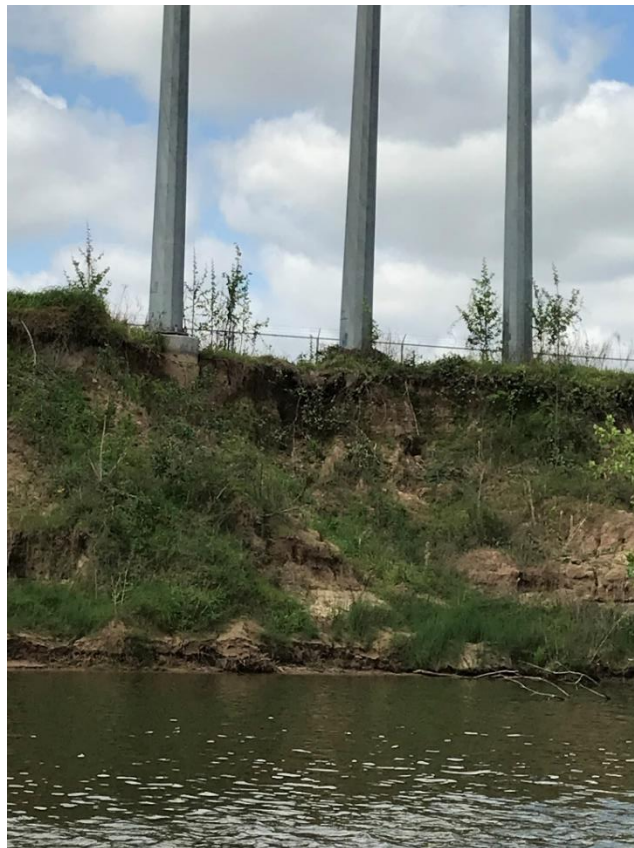
Figure 3: Streambank erosion close to utilities at Mary Rhodes Pump Station
