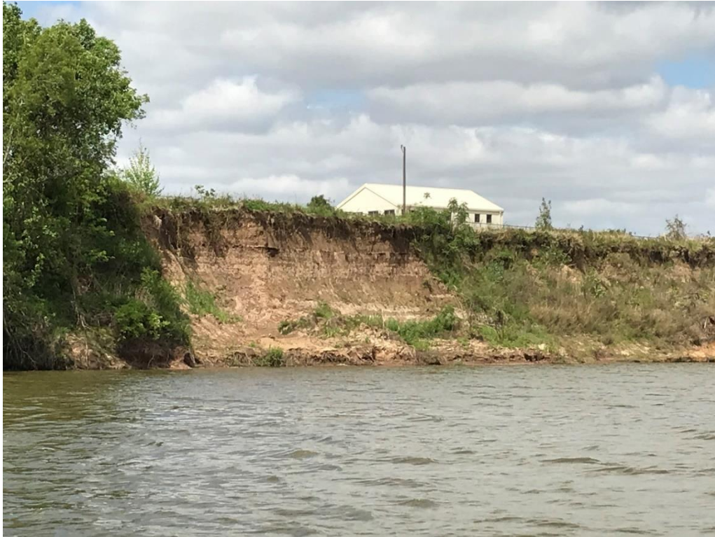
Figure 2: Streambank Erosion at Mary Rhodes Pump Station
