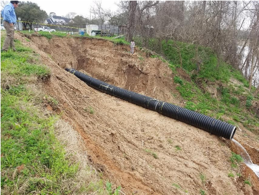
Figure 6: Site conditions as of March 2018 including the failed emergency repair and temporary pipe
