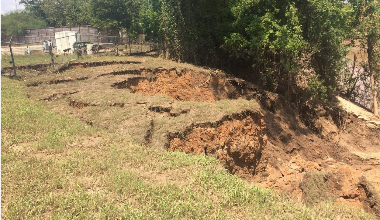
Figure 5: Erosion following Hurricane Harvey
